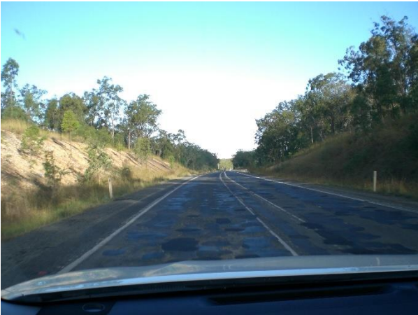
Surface failures and deteriorated ATLM, Lowmead area
