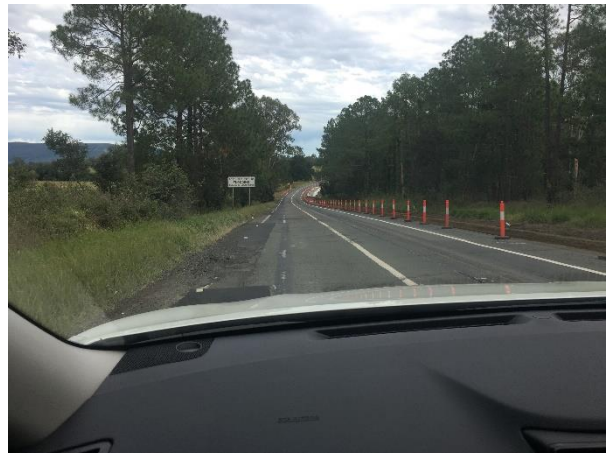
Damage and roadworks on D'Aguilar Highway
