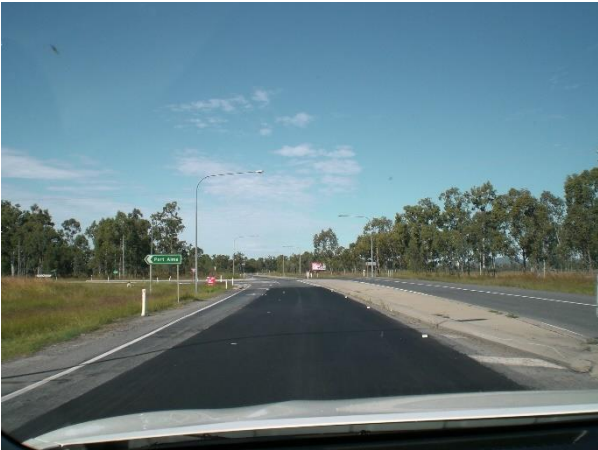
Patched section of road
