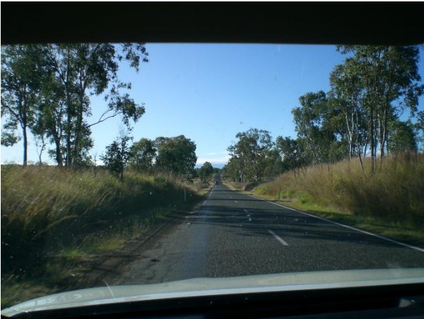
Narrow and surface failures and edge breaks north of Monto
