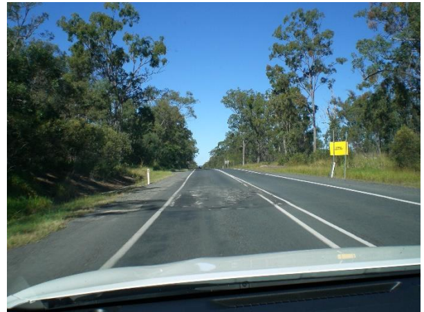
Patchy road surface / surface failures
