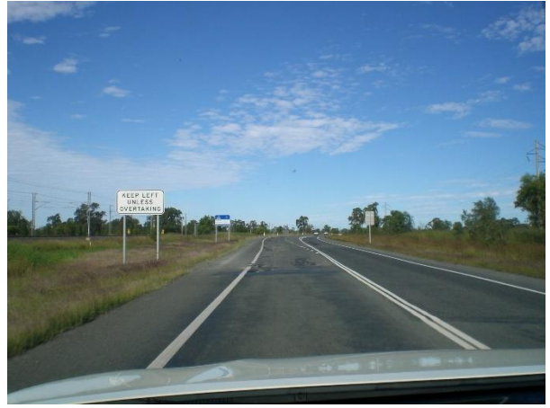
Rough surface and evidence of pavement failures
